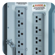
Device adaptors plug into 4x8-way power strips, 2 on each side.
